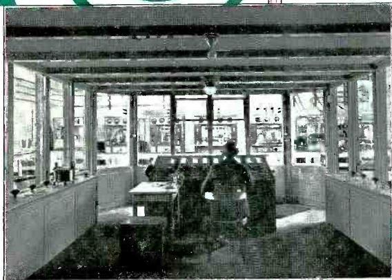
A VIEW IN THE CONTROL-ROOM OF THE PHOI TRANSMITTER
