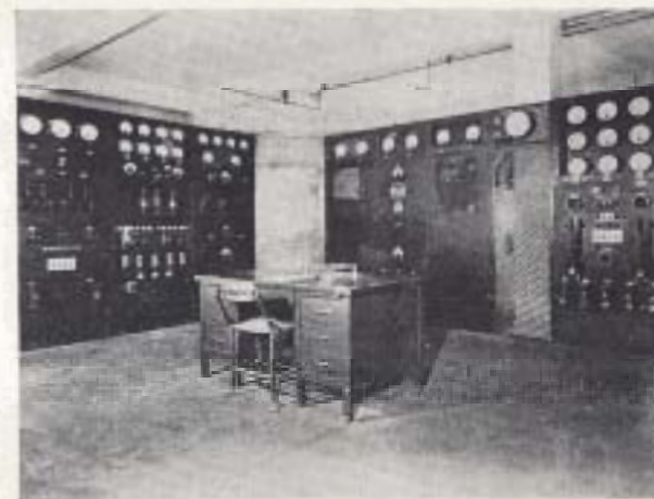
INTERIOR VIEW—TRANSMITTER PANEL
