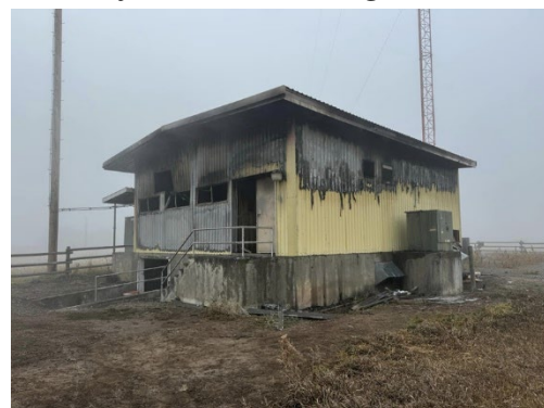
Photo of damaged KOFI transmitter building (KOFI Facebook via Shawn Axelrod)
